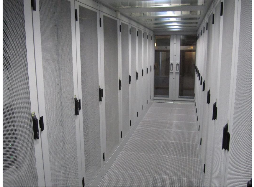
NikhefHousing: a cold aisle
