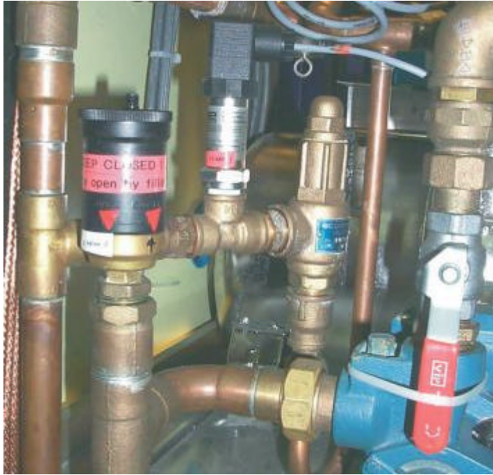
Figure 6.2: Location of the air-bleeding valve
