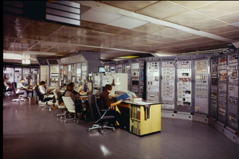
Image: PS control room at CERN
